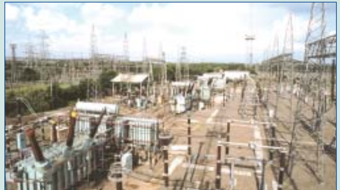
India's first indigenously developed thyristor-controlled series capacitors for improving power flow and system stability in 400kV systems successfully test-commissioned at Ballabgarh
