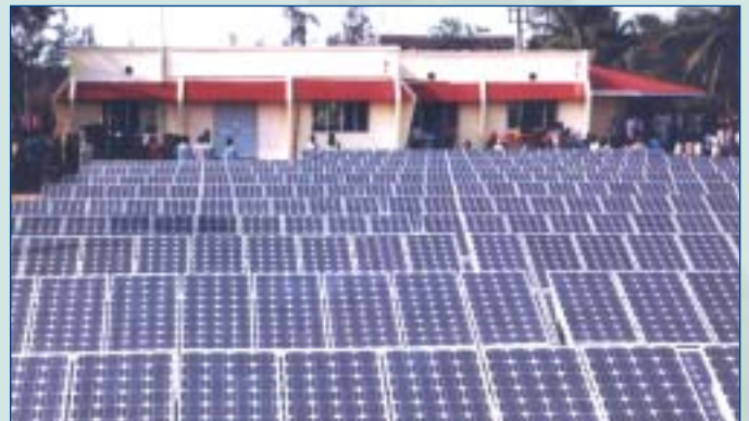
'Stand-Alone' Solar Photovoltaic (SPV) power plant commissioned at Mousuni Island
