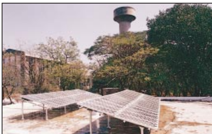
SPV array for pumping water to a 38 m high overhead tank
