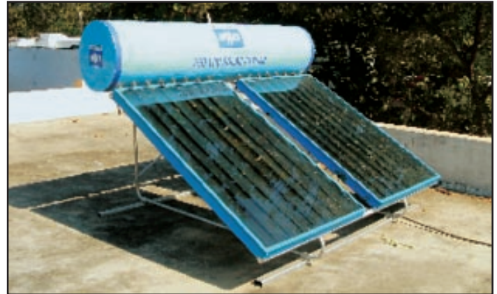
250 LPD Solar Water Heating System
