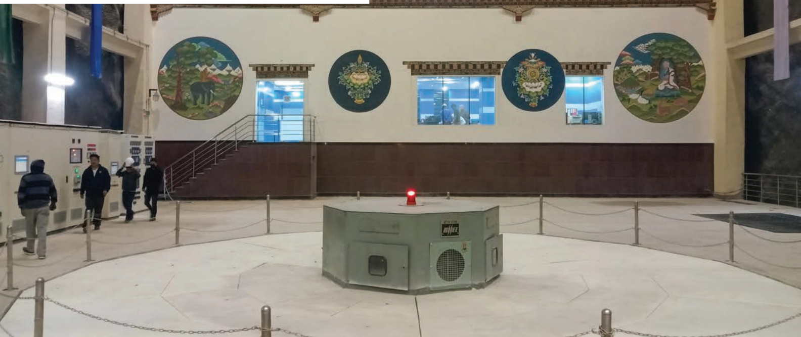
Hydro power plant at Bhutan, 720 MW HEP Mangdechhu designed, manufactured and commissioned by BHEL, was jointly inaugurated by Hon'ble PM (India), Sh. Narendra Modi and Hon'ble PM (Bhutan), Dr. Lotay Tshering in August 2019
