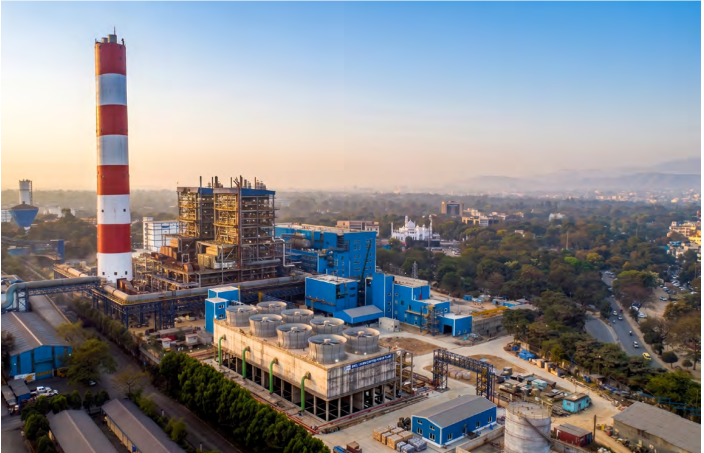
IEL Jamshedpur 1X120 MW Project (First project being executed by BHEL with 100% BFG firing requirements)
