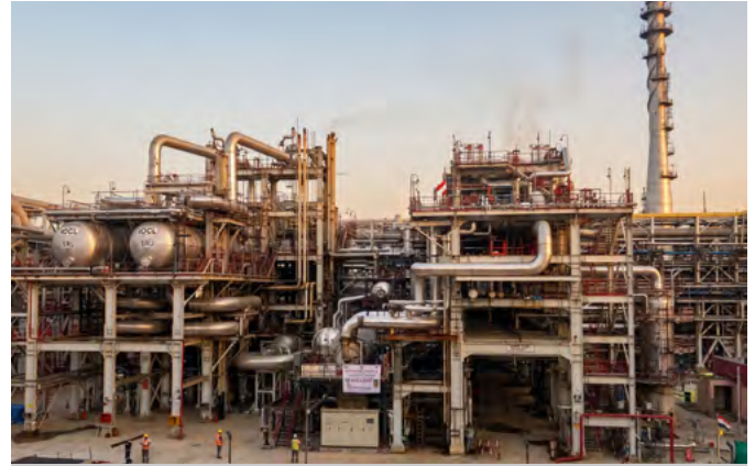
Sulphur Recovery Unit (SRU) package at IOCL Paradip Refinery, Odisha successfully executed by BHEL
