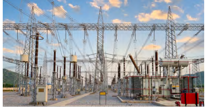
All three substations of 400/200 kV of Neemuch Transmission System were successfully energized
