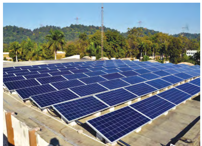
5MW Solar Power Plant at HEEP, Haridwar
